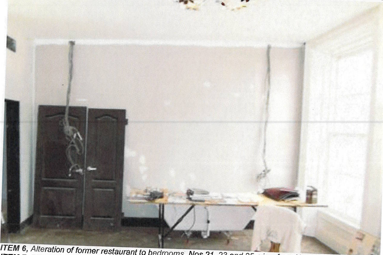
ITEM 6 , Alteration of former restaurant to bedrooms, Nos.21, 23 and 25, view from No.23, June 2005, and ITEM 7 , Filling in of 1970s niches above chimney breast, Nos.21 and 23, June 2005, note modern materials
