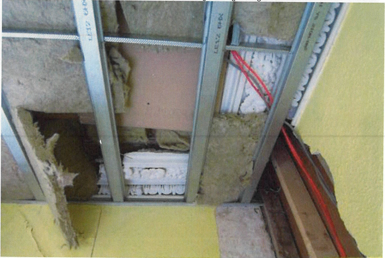
ITEM 1, Banquet Suite, No.27, December 2007, showing fireproof suspended ceiling and existing details retained above
