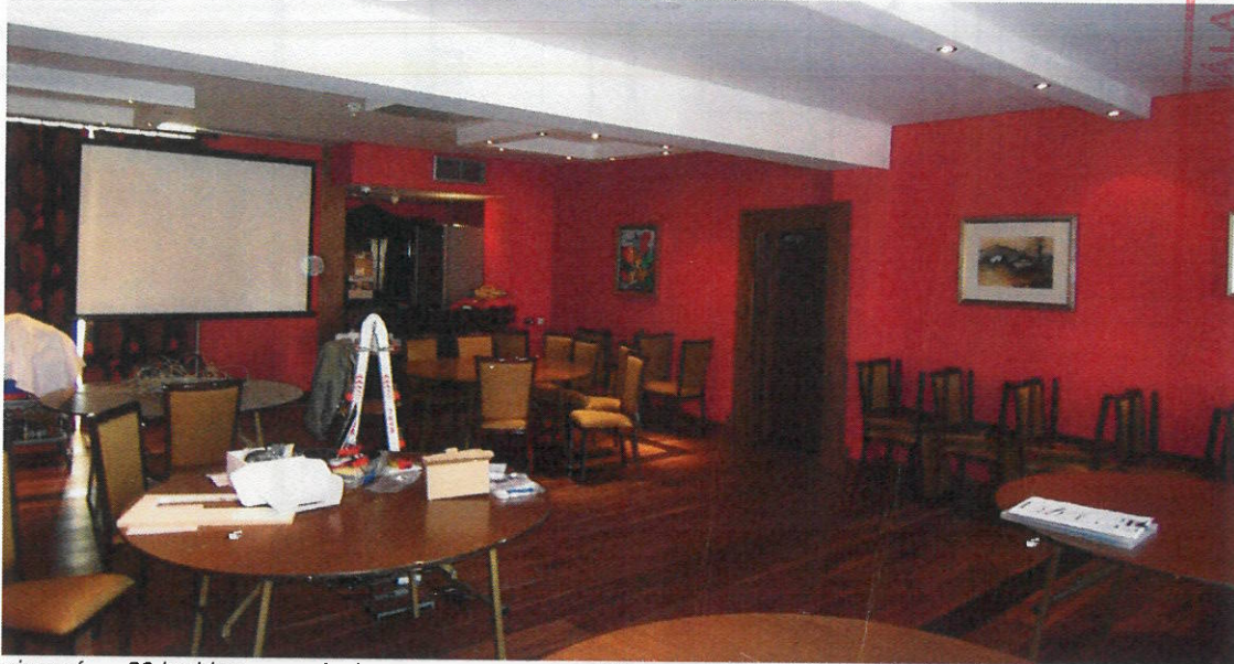
view of no.29 looking towards the recess which could have contained the original stairs
