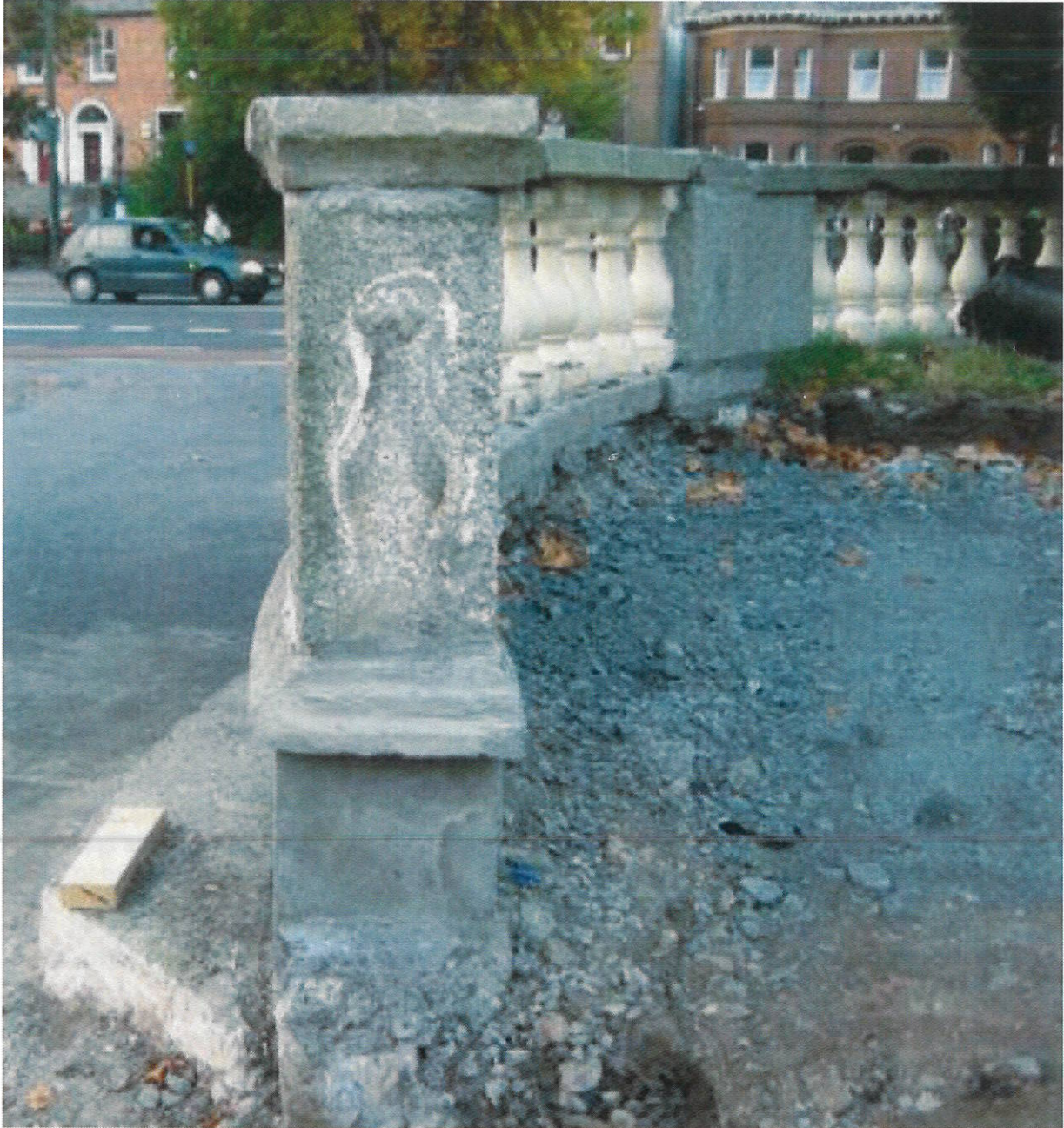
Detail of the damaged section of the balustrade
