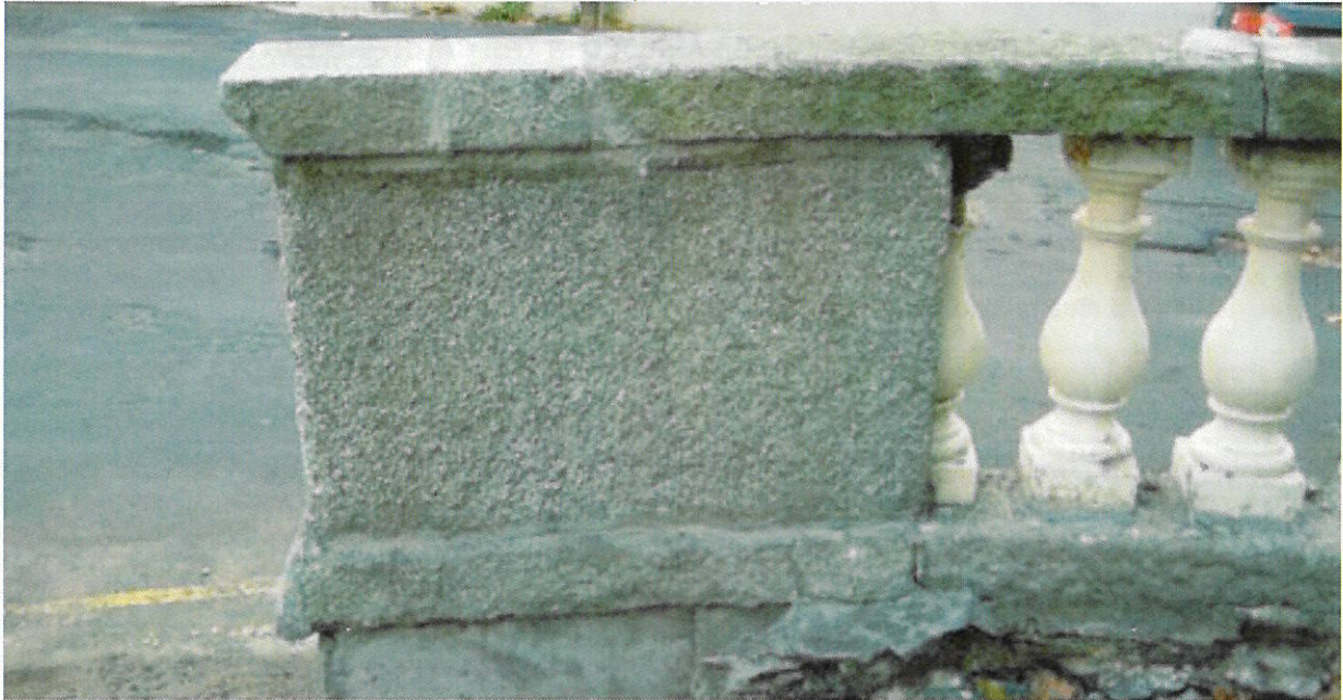
view of present end pier (from inside), concrete base repair visible
