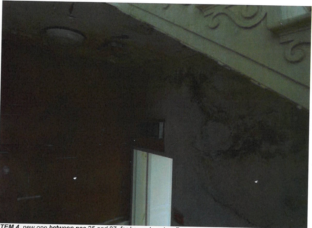
ITEM 4 , new ope between nos.25 and 27, for house keeping, December 2006, note wall condition
