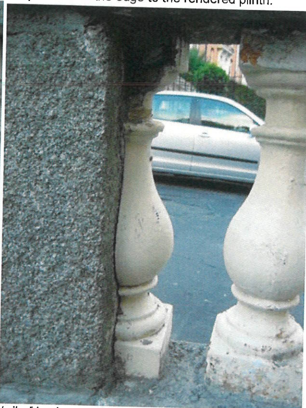
detail of broken cast iron balustrade, to be used for new
