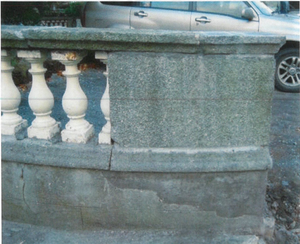
view of present end pier (from outside), concrete base repair visible
